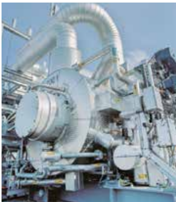
Air conditioning & compressors
